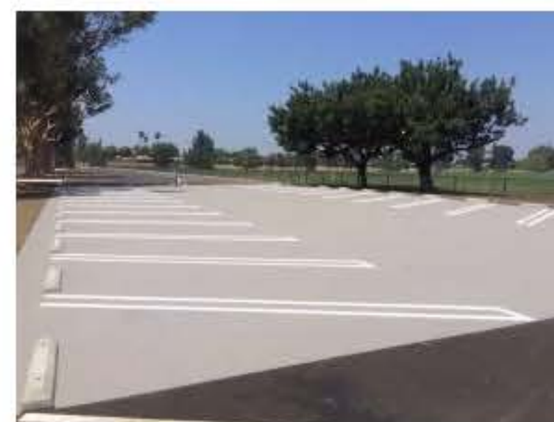
A parking covered in CoolSeal was on average 10 degrees cooler than conventional asphalt. (Photo courtesy of the City of Los Angeles)
